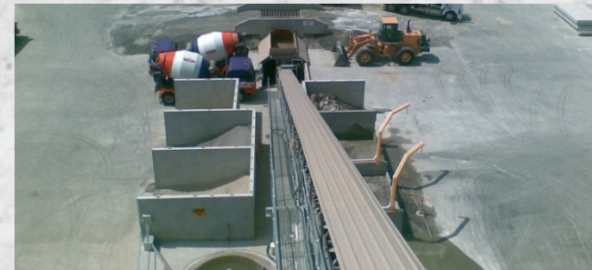
Concrete Plant Bins
